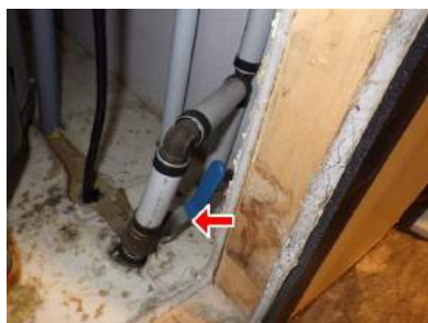
5.0 Main Water Valve
