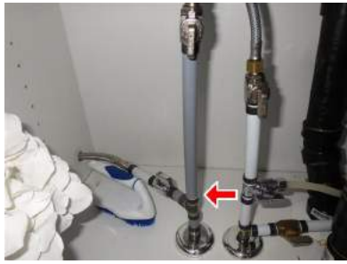
5.3 PolyB with Copper Fittings
