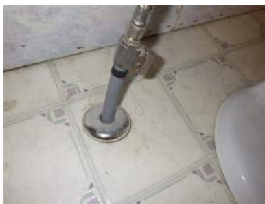
5.3 PolyB with Copper Fittings
