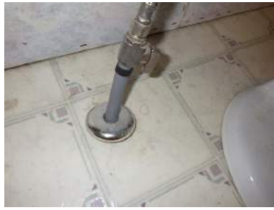
5.3 PolyB with Copper Fittings
